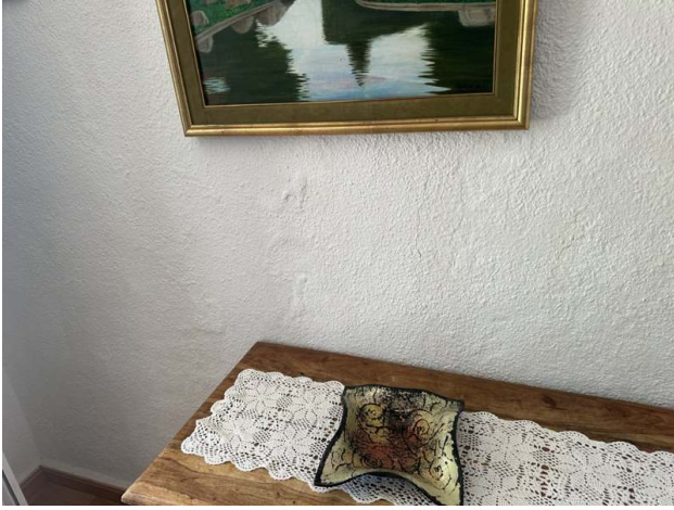
Staircase junction: water getting into the ground-floor bedroom.
