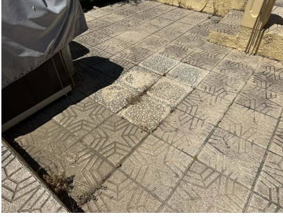
Terrace: damaged and lifted tiles across the property.
