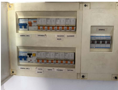
Main consumer unit (fuse box).
