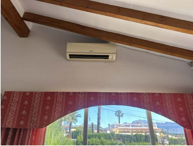
A/C units on the main terrace, both aged.
