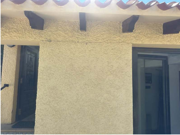
Render cracks on the exterior façade.
