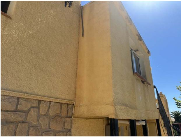
Master bedroom extension: corrosion and water ingress.
